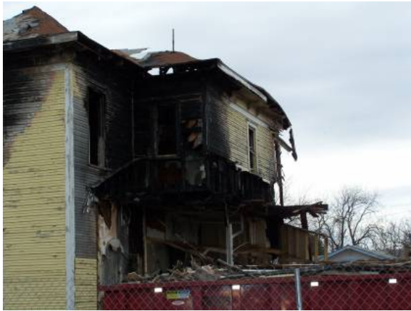
Fire damage before repair
